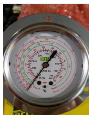
Example of empty (loss of refrigerant)
