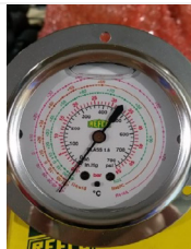
Example of empty (loss of refrigerant)
