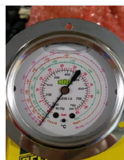
Example of empty (loss of refrigerant)
